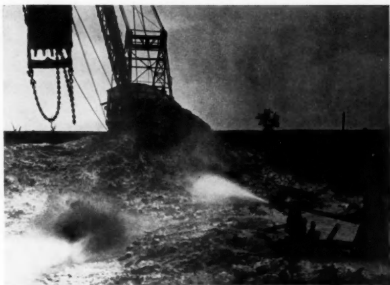
A DRAGLINE DREDGE transports uranium-bearing ore to site where HIGH-PRESSURE MONITORS wash it down into sludge. The sludge is carried by pipeline to the phosphate concentrating plant. (Virginia-Carolina Corporation operation near Bartow, Florida.)
